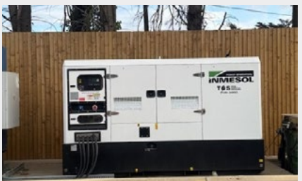
New Generator & Acoustic Fencing
